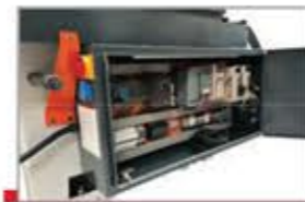
Elektrik paneli Electric panel
