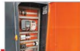
Elektrik Panosu Electric Panel
