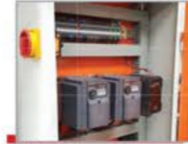
Elektrik Panosu Electric Panel
