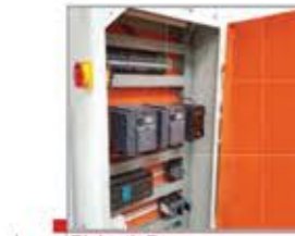
Elektrik Panosu Electric Panel
