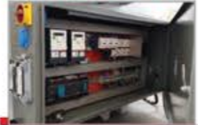
Elektrik panosu Electric Panel
