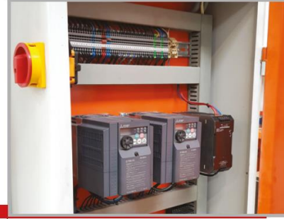
Elektrik Panosu Electric Panel
