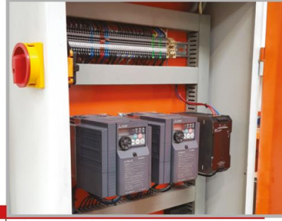
Elektrik Panosu Electric Panel
