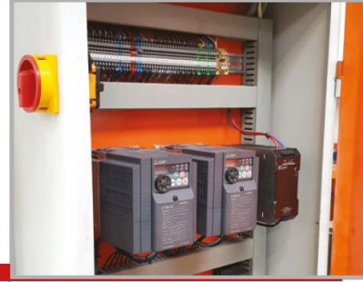
Elektrik Panosu Electric Panel
